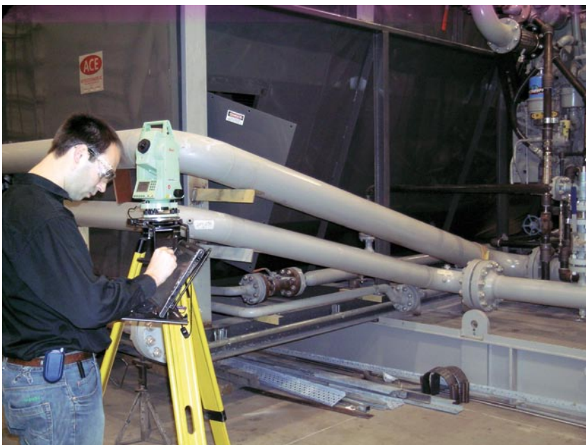
Figure 1. CADWorx fieldPipe in operation with the tripod mounted Leica Total Station and Leica fieldGear.
